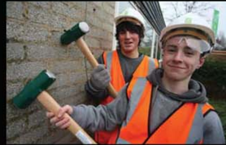
Countesthorpe Community College students Will Attfield (front) and Lewis Sreaton (rear) preparing to demolish the bungalow.
